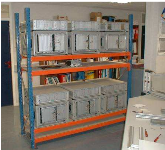
Figure 6: View of the rack to be used in the 30-m backend room.
